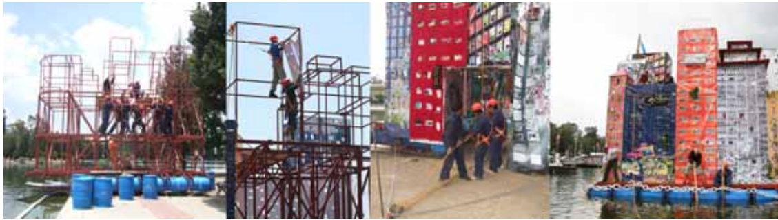
stages in the installation of the floating city (assembling the structure, mounting the decorations, pulling the city in the water, and in its final position)
